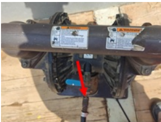
Disconnected hose end connection
