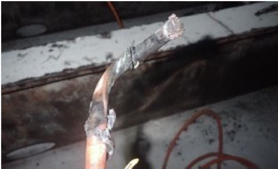
Photo of fire damaged welding cable
