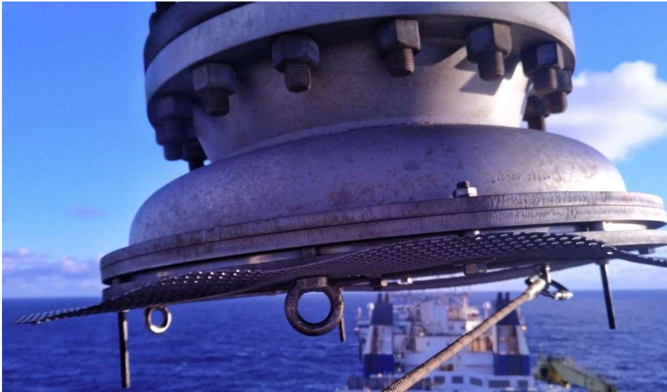
Figure 3: Atmospheric vent line after the lid had fallen down
