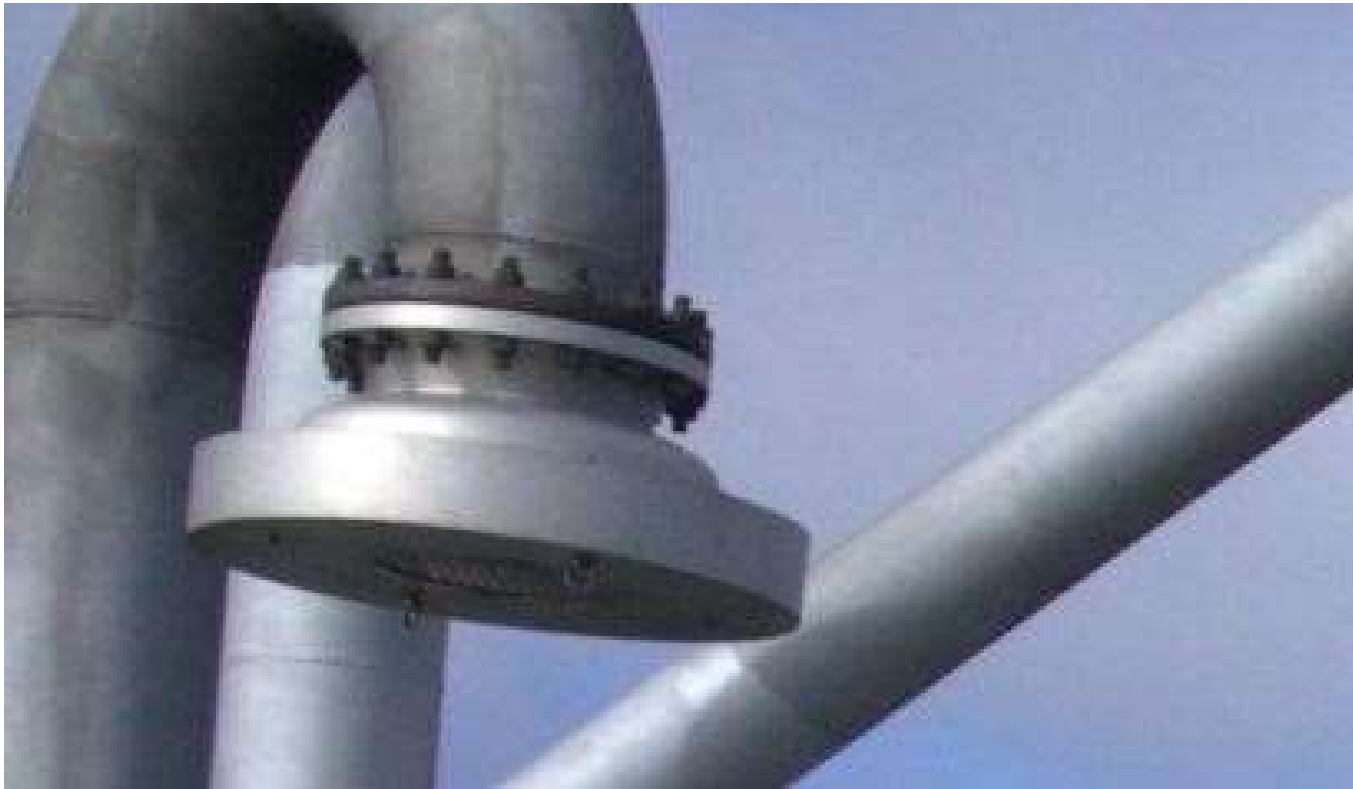
Figure 1: Lid while installed on the atmospheric vent line
