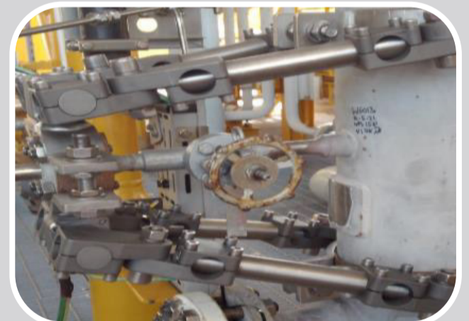
Event 2 – Repaired spool with bracing from end flange to main line to support small bore piping
