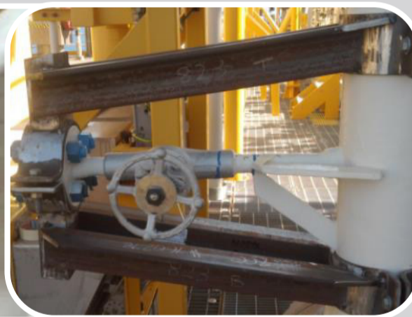
Event 1 – Permanent bracing (unpainted in photo) installed on straight small bore piping on gas booster compressor relief lines
