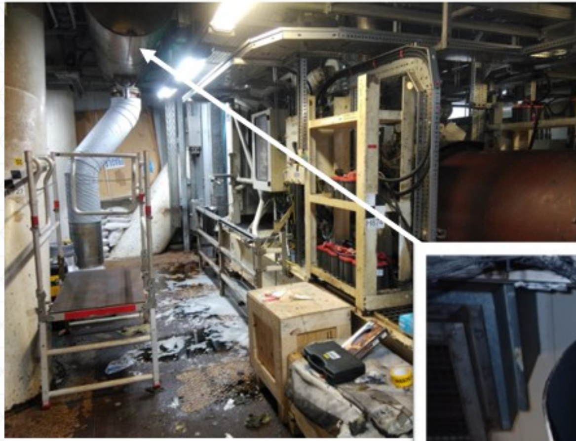
Diesel engine compartment with failed silence / spark arrestor
