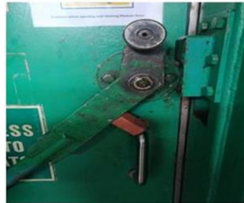
Door lock handle has now been fixed providing protection and stopping the door lock handle from swinging free.
