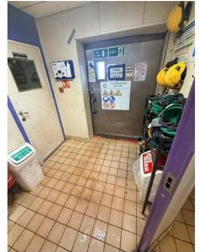
External accommodation door contributed causing a pressure change.
